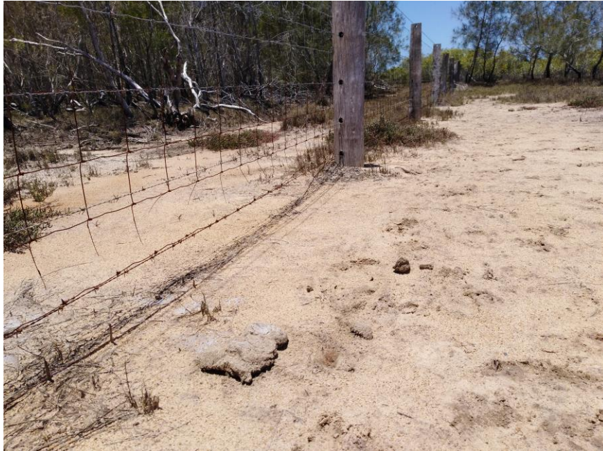
Figure 53. Round Hill fence after 3yrs exposed to tidal wetland soils. Corrosion compromises the integrity of the base of the fence, and potentially permitting feral pig access to the wetland. Fencing maintenance will be on-going in coastal areas subject to harsh marine conditions, but is presumably costly.
